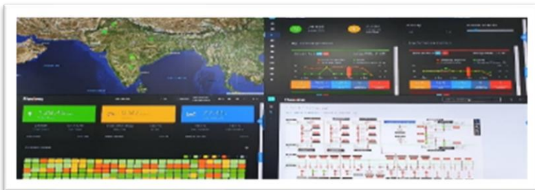
Centralised Control Room for Proactive Asset Management
